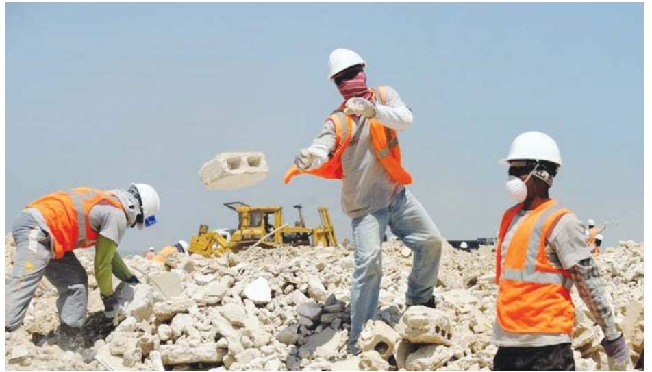
PHS, a Haitian American firm, removes rubble at the Truitier landfill in Port-au-Prince, Haiti. Photo Credit: Kendra Helmer
